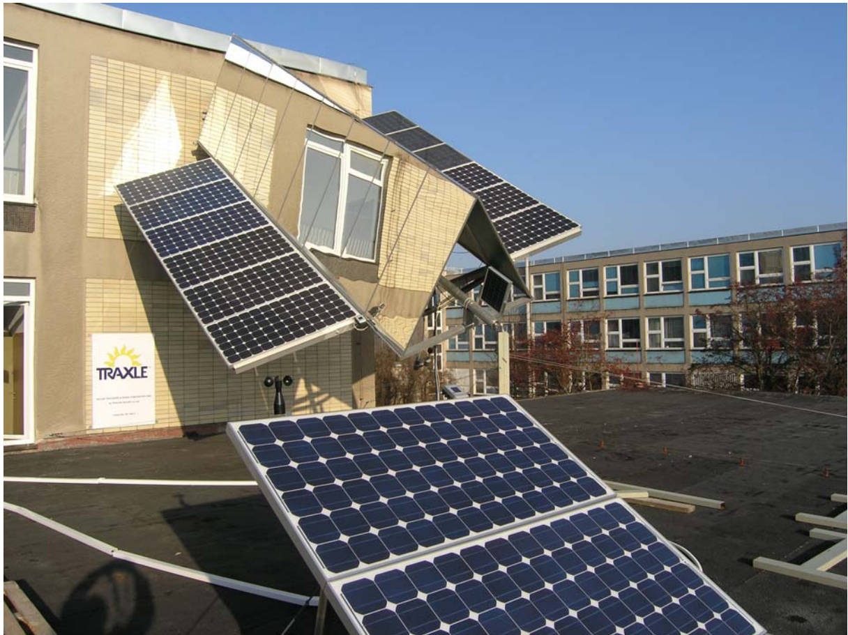
Fig. 2. Photograph of the tracking ridge concentrator and a part of the fixed PV system
